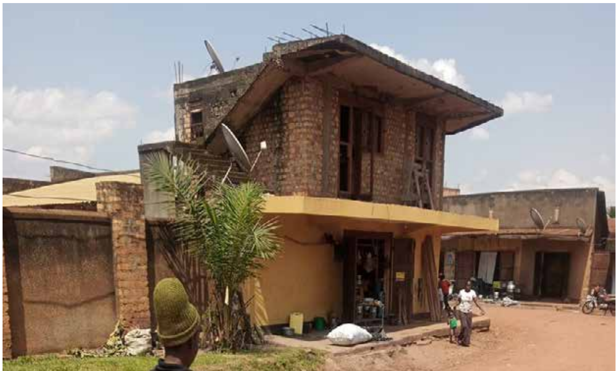
Figure 4: Critical site in Mityana MC with deflecting 1.8m & 2m cantilever slab panels
