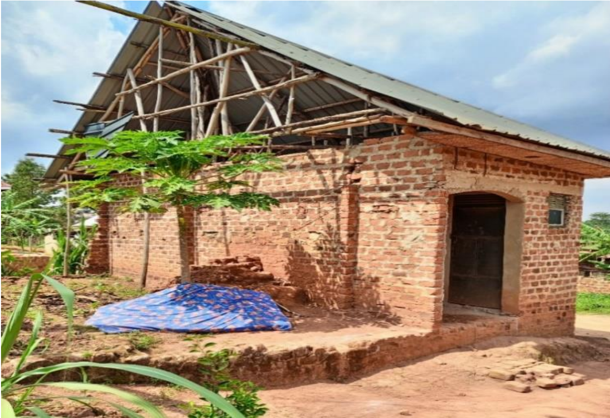
Figure 5: A Partially occupied building, the roof trusses are made of eucalyptus poles.
