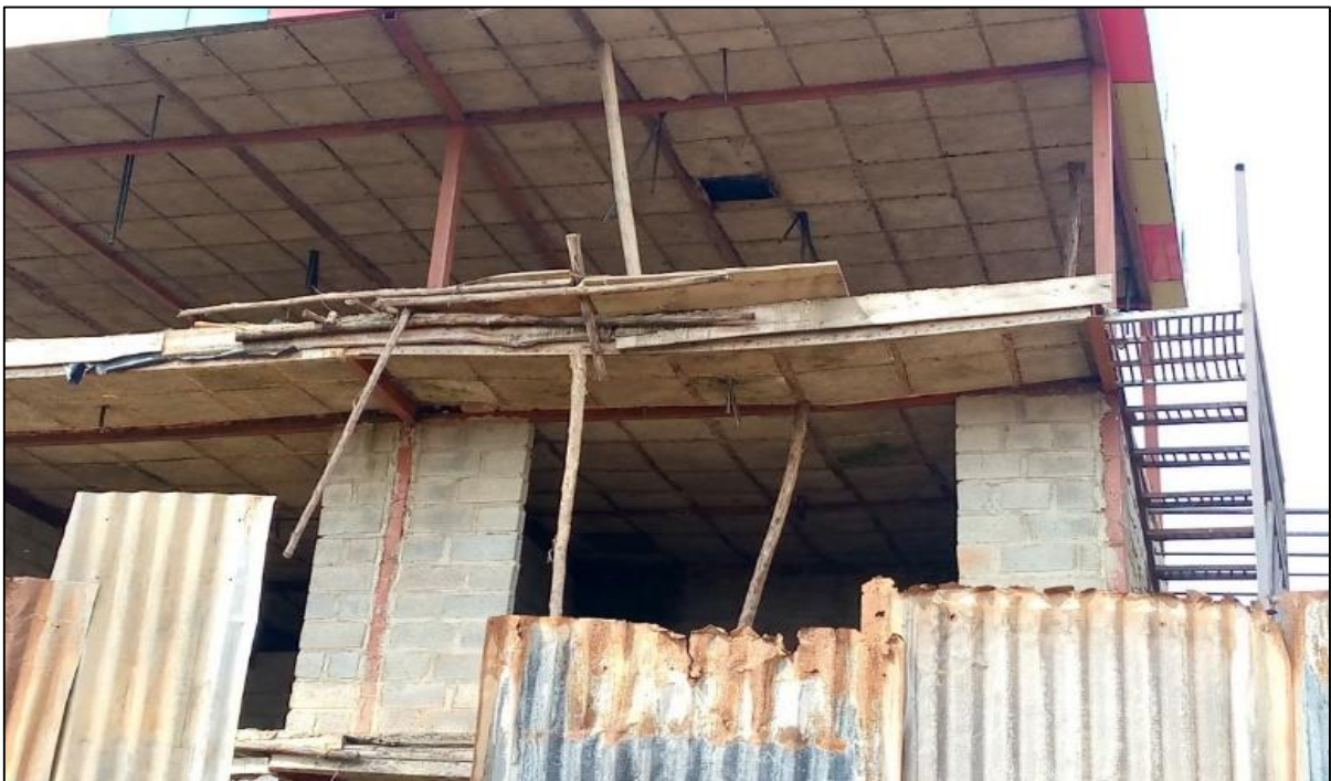
Figure 32: Dormant STC structure with high risk of collapse in Namugongo, Bulooli Village
