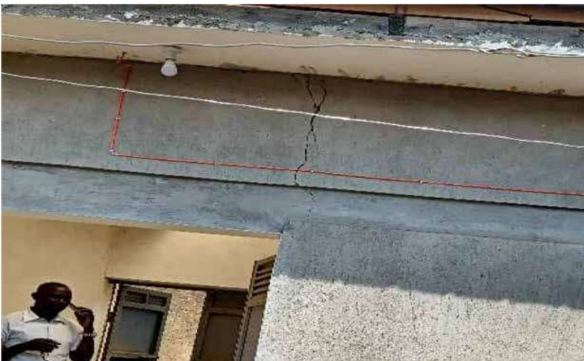
Figure 2: Building in Apac MC with cracks above ring-beam level
