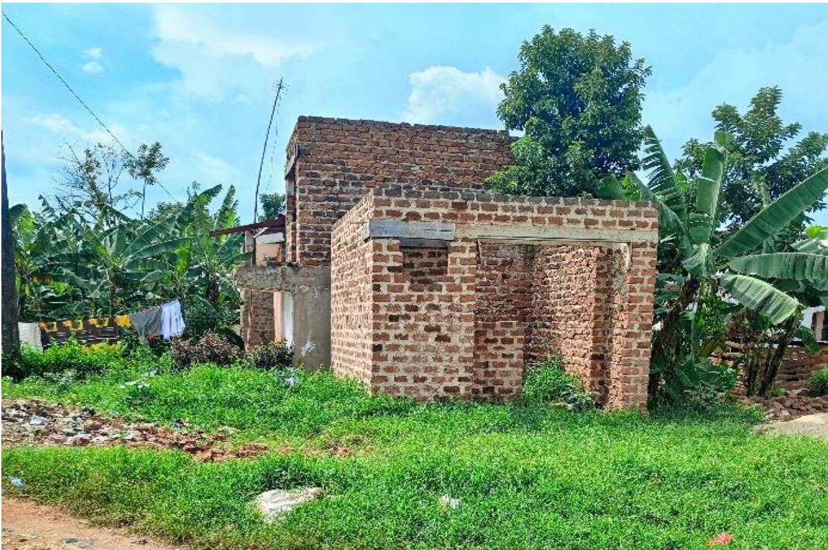
Figure 6: A non - Conventional structure, no reinforcement columns on the first floor
