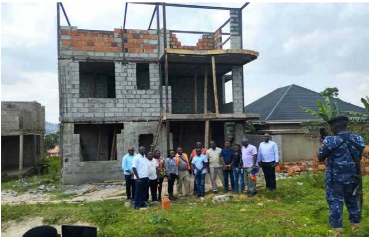
Figure 98: STC Technical committee members in a field visit of the prohibited construction
