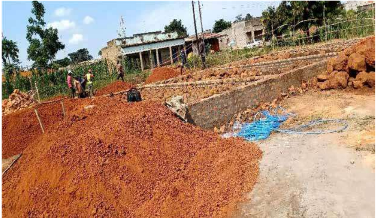
Figure 3: Construction site in Apac; no safety measures; backfill not compacted
