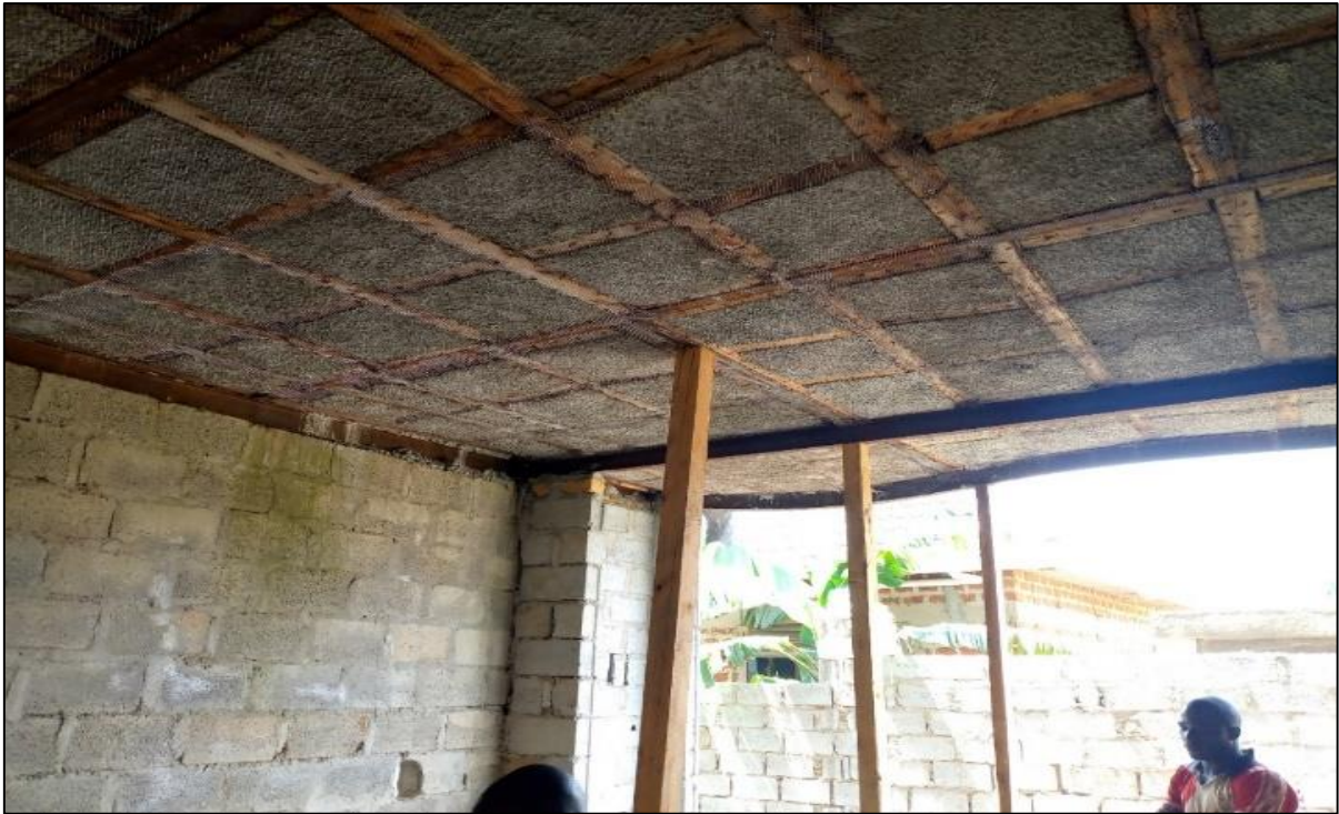
Figure 31: Failing Steel Timber Concrete (STC) Composite slab propped with timber poles
