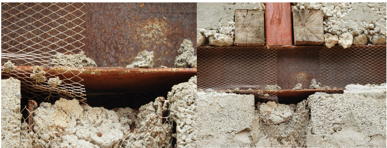
Figure 2-17: No contact between beam and its supposed lower column section
