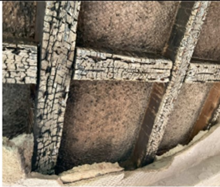
Figure 3-15: Charred Timber of STC floor system after the fire
