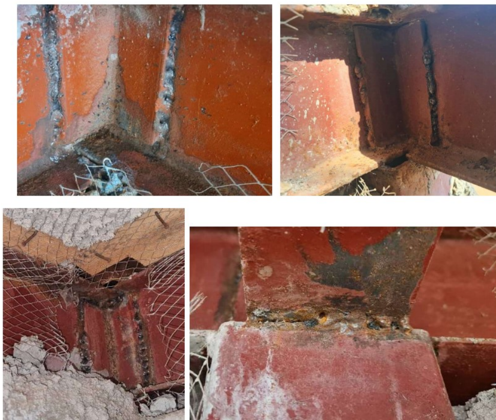
Figure 3-10: No fusion between the base metal and the angle bar
