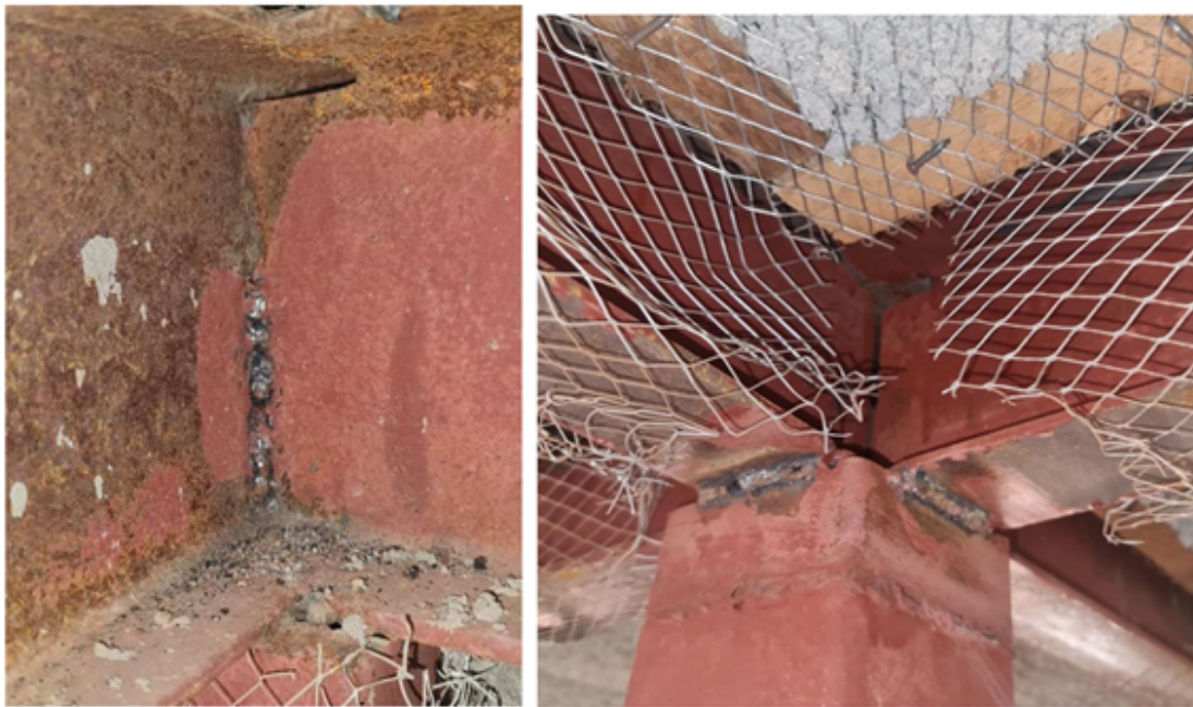
Figure 3-9: Poorly welded joints with inconsistency in weld profile
