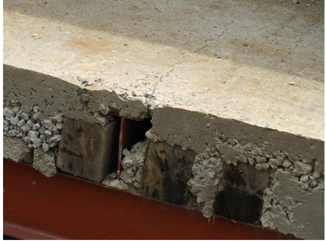
b) Crack along the flange line
