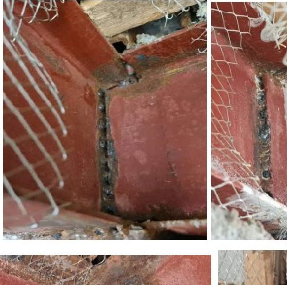
Figure 7-4: School in Nansana with welds showing lack of proper fusion at joints
