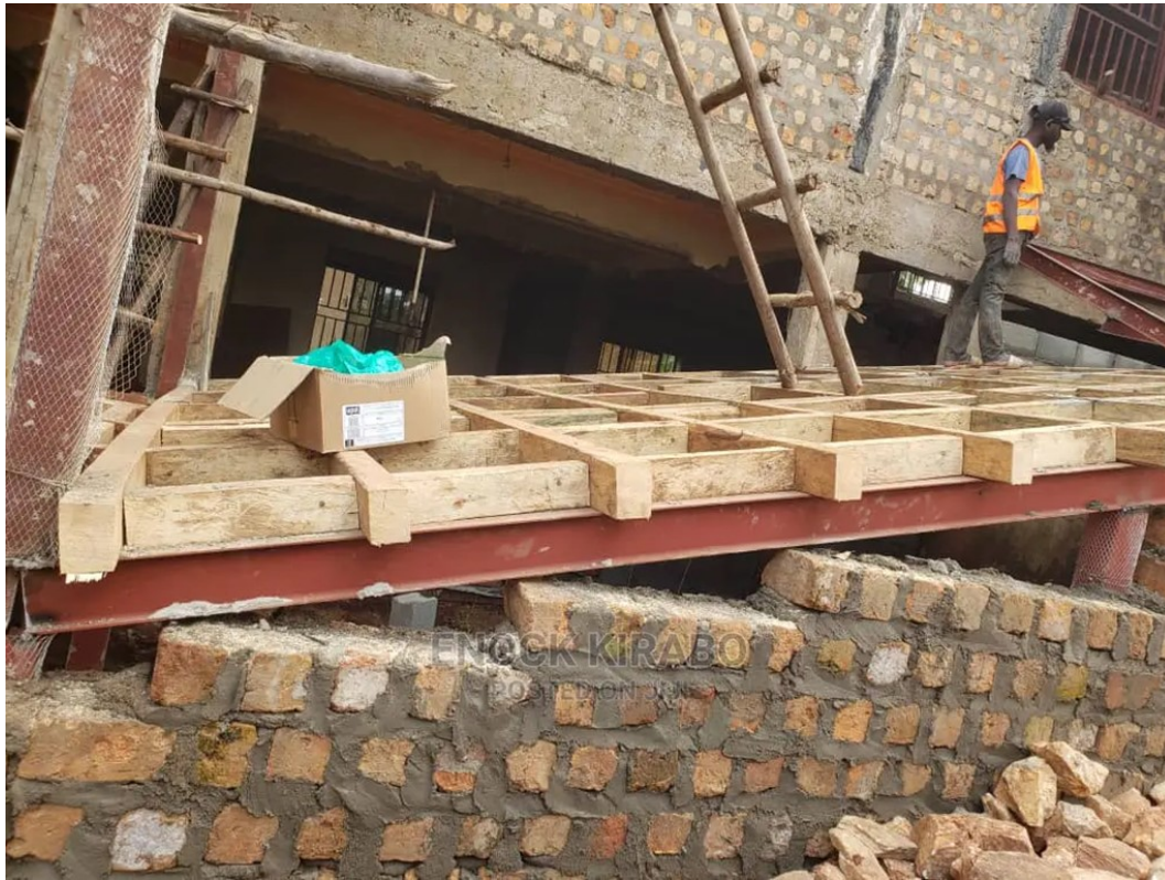
Figure 3-8: Timber framework simply placed on top of the steel beams (Credit: Enock Kirabo)
