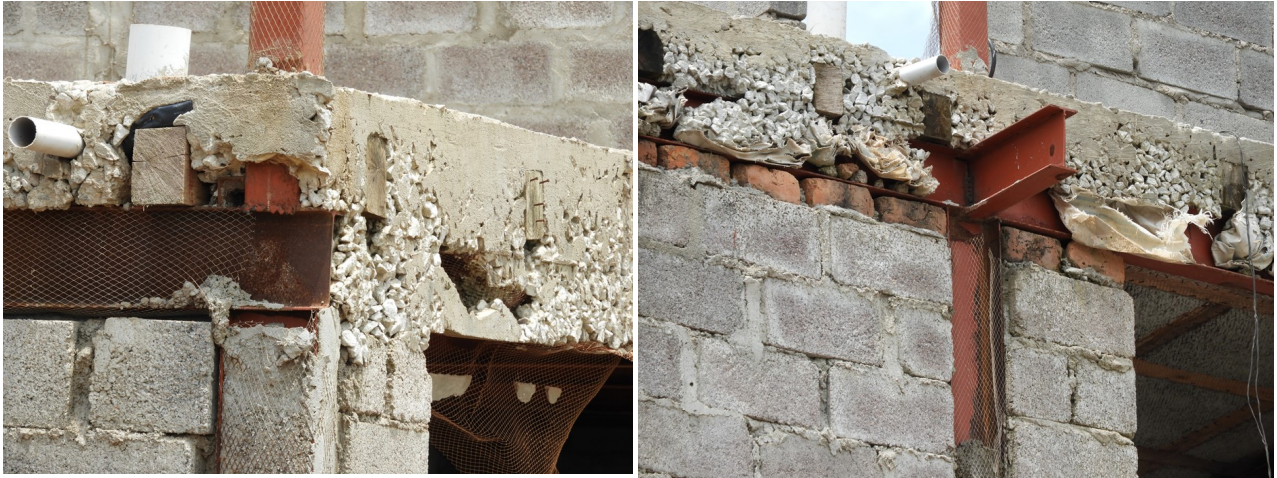
Figure 2-9: Concrete honey combing
