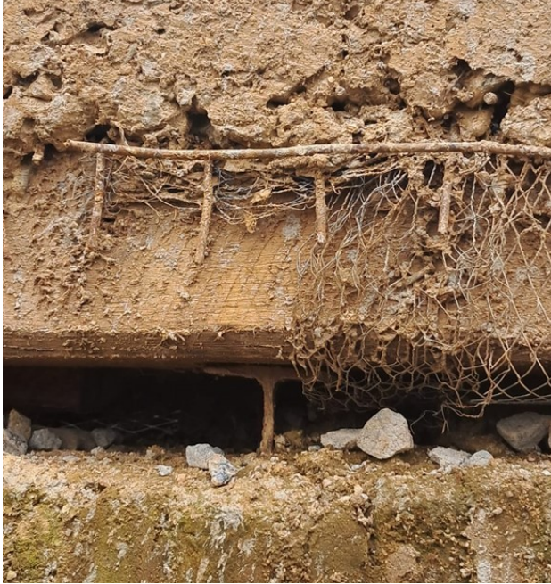
(a) Buckled beam web
