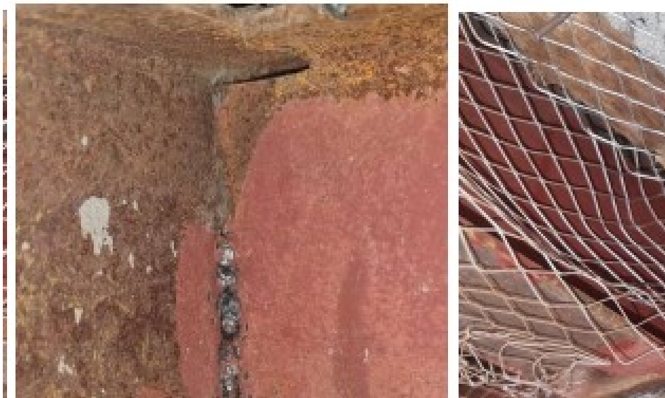
Figure 7-2: School in Nansana with little-to-no weld connection of the steel sections
