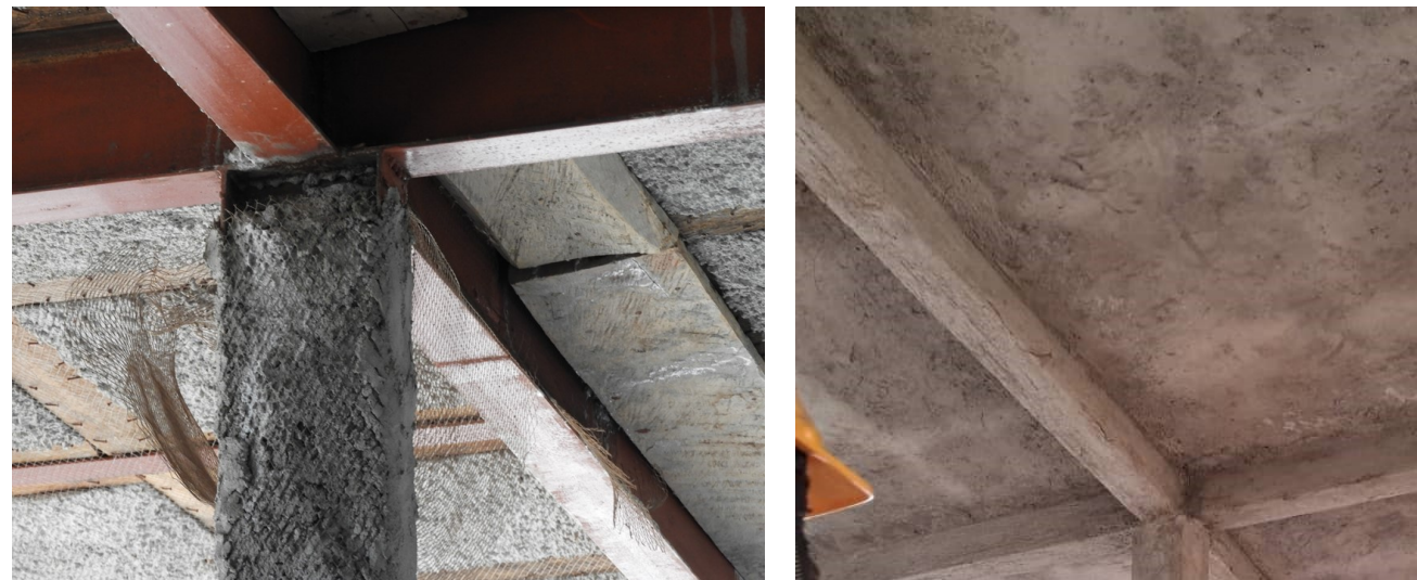
Figure 2-11: Metal lathe layer filled and eventually plastered to encase the steel sections
