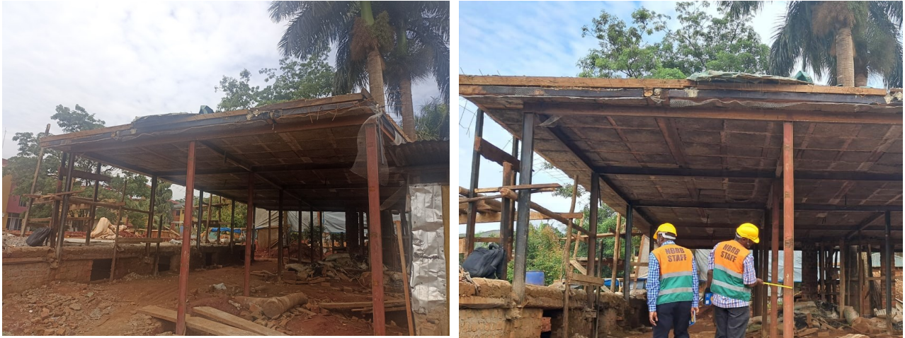
Figure 2-3: Storage block at a hotel
