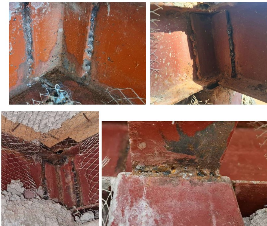
Figure 7-17: No fusion between the base metal and the angle iron
