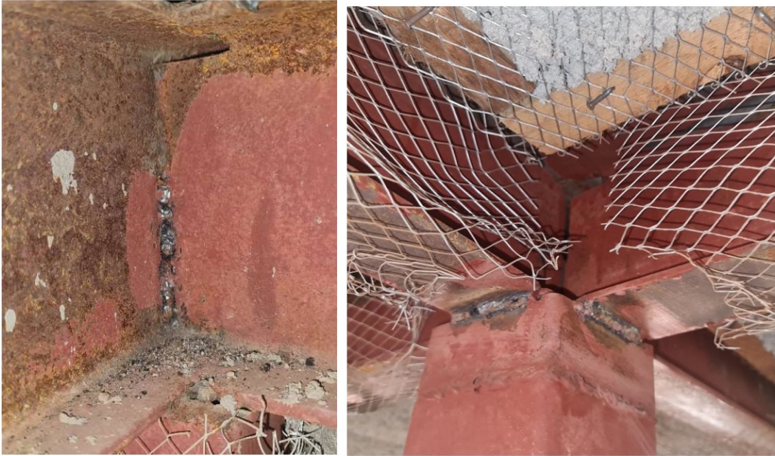
Figure 7-16: Poorly welded joints with inconsistency in weld profile.
