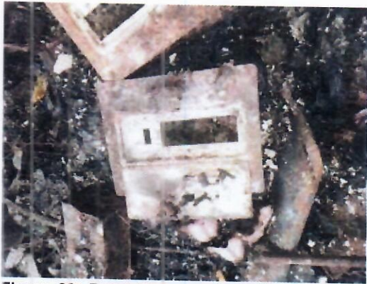
Figure 26: Burnt Consumer's Units of Ground Floor of Northern Wing of Main Building
