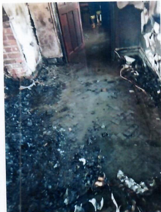
Figure 7: Hot Water from Fire Truck in Corridor of Southern Wing of Main Building
