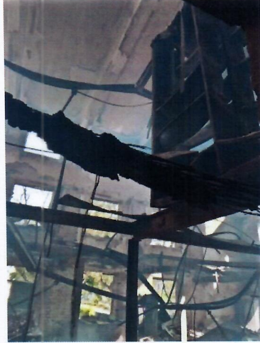
Figure 11: Burnt Out First Floor, Southern Wing of Main Building with Hanging Bookshelf
