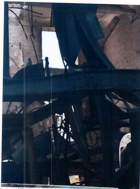
Figure 17: Burnt Staircase of First Floor, Northern Main Building
