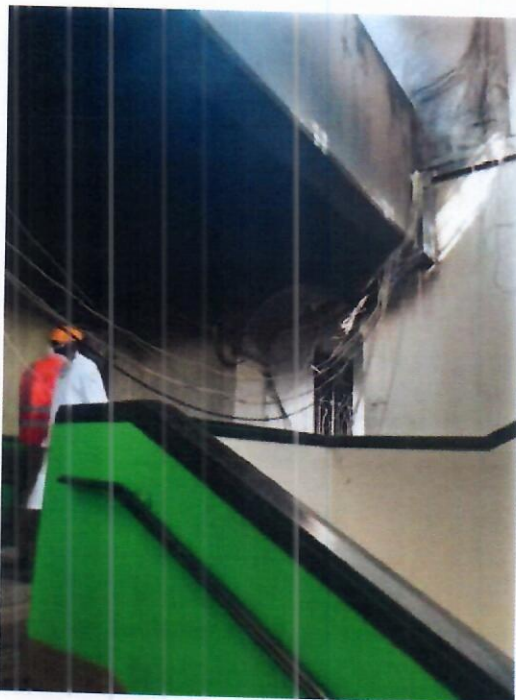
Figure 19: Exposed Wires from Burnt PVC Trunking in Corridor of First Floor of Main Building
