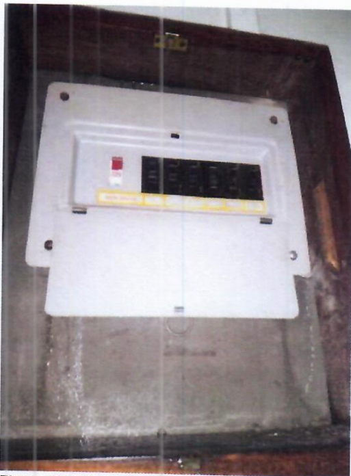
Figure 28: Consumer's Unit in Common Room on Ground Floor, Southern Wing of Main Building
