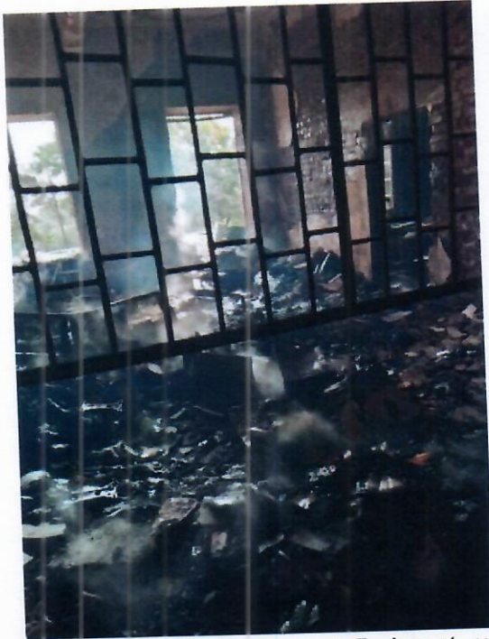
Figure 8: Burnt Furniture and Equipment on Ground Floor Office, Southern Wing of Main Building
