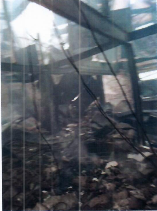
Figure 10: Smoke Going through Open Roof of Northern Wing of Main Building
