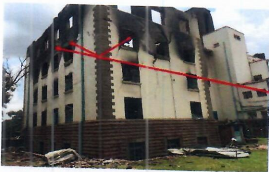
Figure 16: Soot Deposition Pattern in Windows on First Floor of Northern Wing of Main Building
