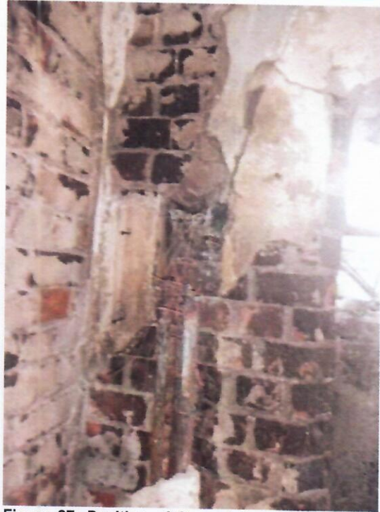
Figure 27: Position of Second Burnt Consumer's Units on Ground Floor of Northern Wing of Main Building
