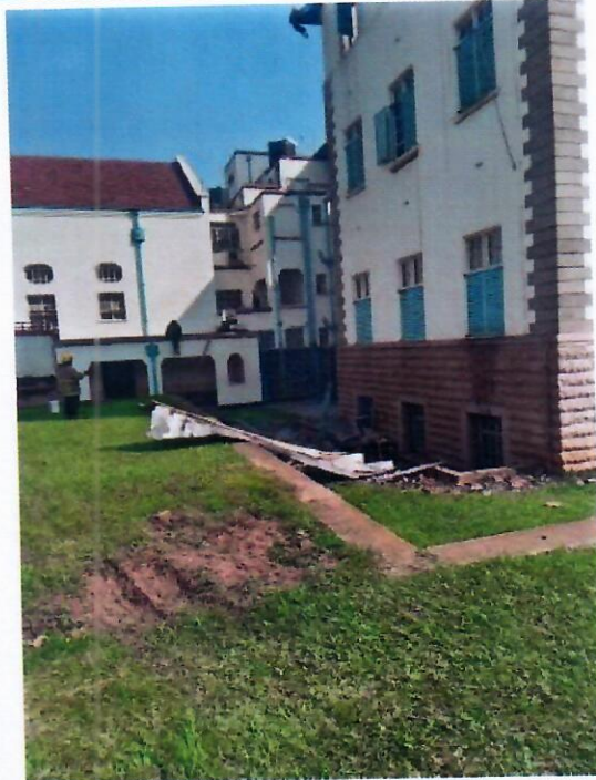
Figure 5: Debris Behind Southern Wing of Main Building
