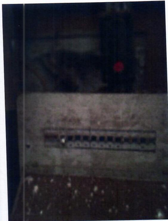
Figure 33: Consumer's Unit 2 in Ceiling of Stage of Main Hall
