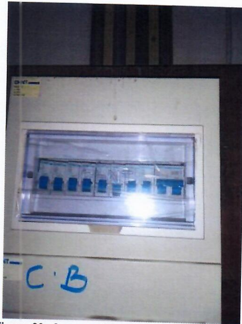
Figure 30: Consumer's Unit for Sockets on First Floor of Main Building
