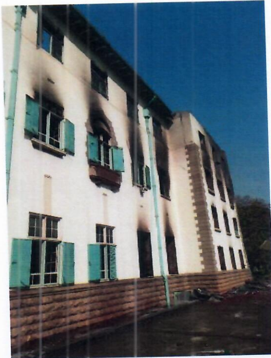
Figure 2: Front of Northern Wing of Main Building Showing with Smoke on Windows
