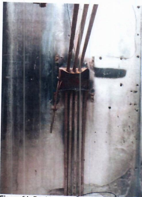
Figure 31: Position of Burnt Consumer's Units for Lights and Sockets on Second Floor of Main Building
