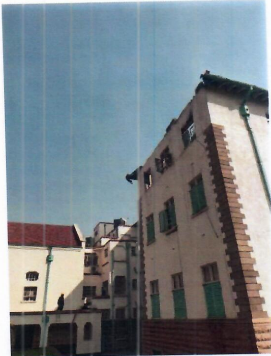
Figure 4: Back of Southern Wing of Main Building with Burnt Windows on Second Floor and No Roof
