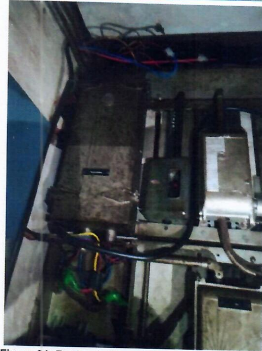
Figure 21: Busbar in Power Room of Main Building
